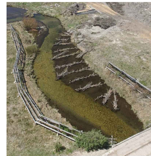
ABOVE: 6 MONTHS POST-CONSTRUCTION; POST LINE WILLOW-WEAVE FENCES WITH FINE SEDIMENT DEPOSITION (BIG SPRINGS CREEK, ID)
