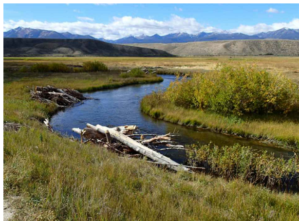
ABOVE: IMMEDIATELY POST-CONSTRUCTION; SMALL WOODY DEBRIS STRUCTURE WITH LARGE WOODY MATERIAL INCORPORATED (BIG SPRINGS CREEK, ID)
