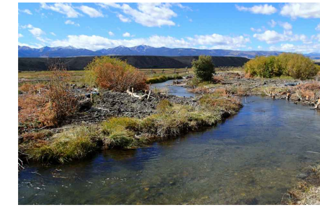
ABOVE: BANK FILL WITH WETLAND SOD BANK IMMEDIATELY AFTER CONSTRUCTION (BIG SPRINGS CREEK, ID)
