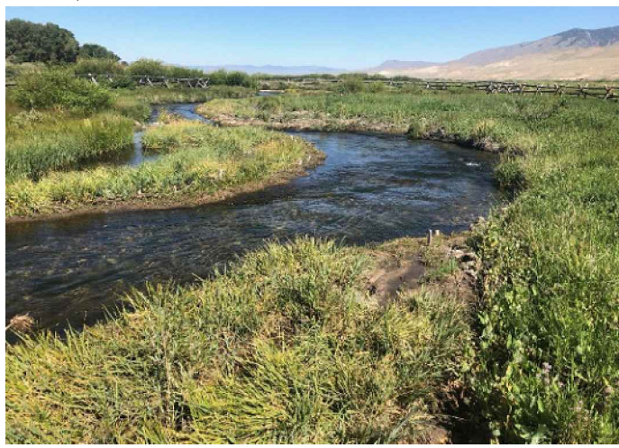
BELOW: POST-CONSTRUCTION; BANK FILL WITH FESL WITH ALCOVE (BIG SPRINGS CREEK, ID)
