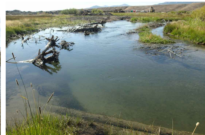
ABOVE: 1-YEAR POST-CONSTRUCTION; LARGE WOODY DEBRIS HABITAT STRUCTURE (BIG SPRINGS CREEK, ID)
